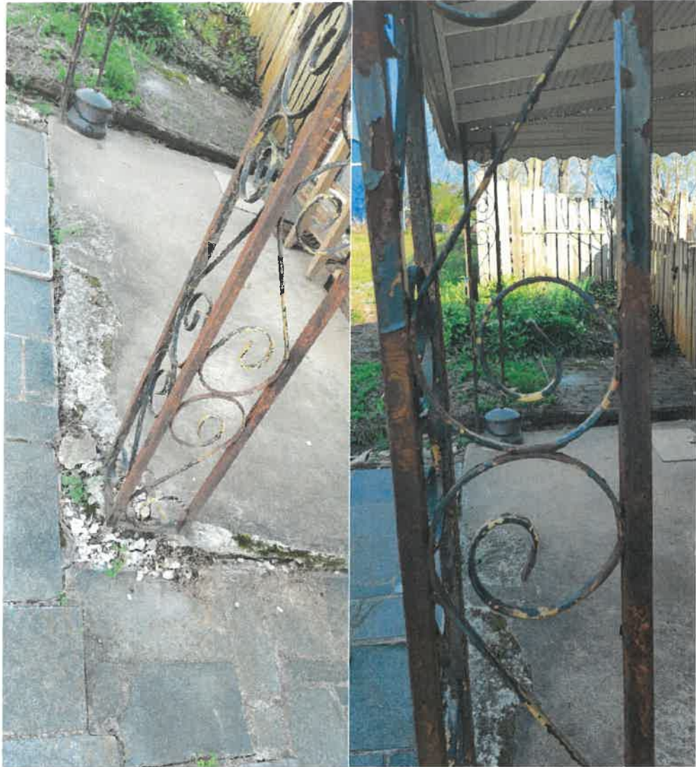
Figures 3 and 4: Deteriorating awning supports and concrete patio
